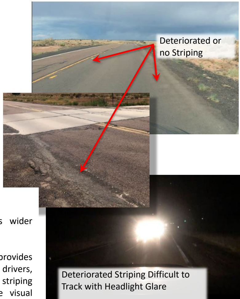
Figure 9 – Pavement Marking Issues
